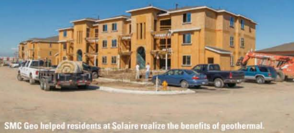
SMC Geo helped residents at Solaire realize the benefits of geothermal.
